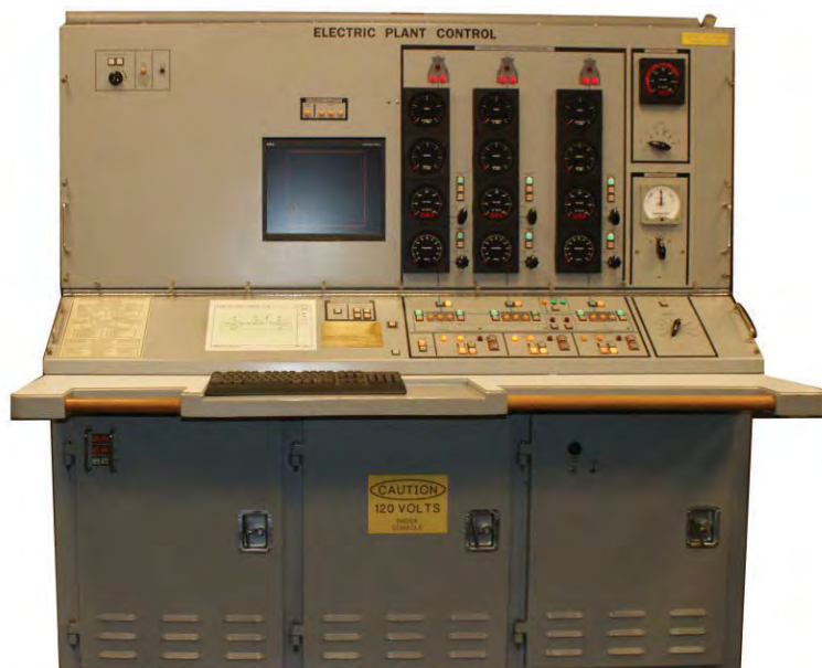
Figure 6-28 — Electrical plant control console.
