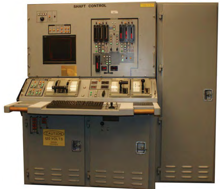
Figure 6-30 — Shaft control unit.
